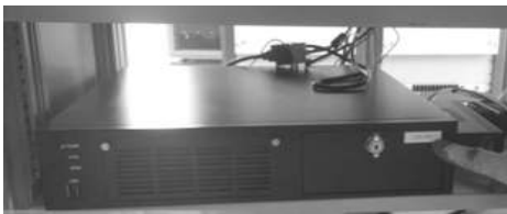
< RCMS Client 설치 >
